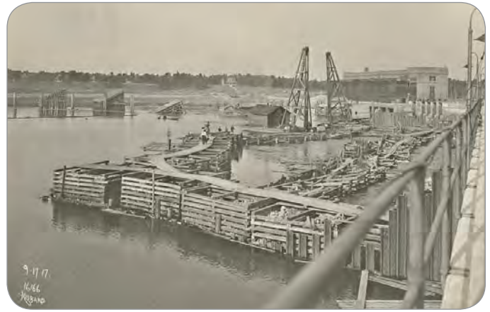
Coon Rapids Dam under reconstruction due to ice dam damage Sept. 17, 1917. Source: Anoka County Historical Society
